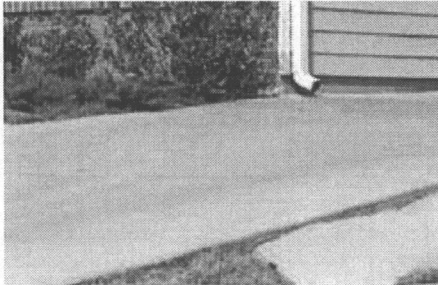
A directly connected roof drain
